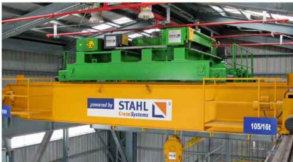
Explosion-protected wire rope hoists in twin design with auxiliary hoist facilitate compressor maintenance in a hydrogen liquefaction plant.
